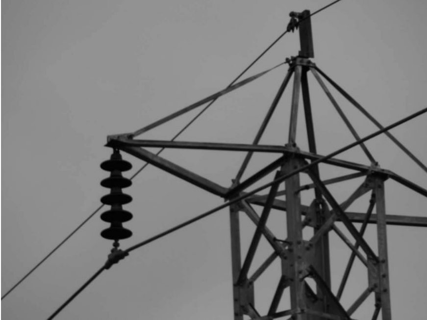
Figure 3.11 Insulator Attachment to Lattice Tower.
