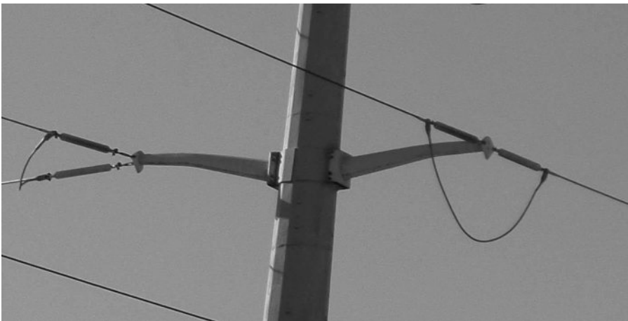
Figure 3.13 Insulator Attachment to Steel Pole.
