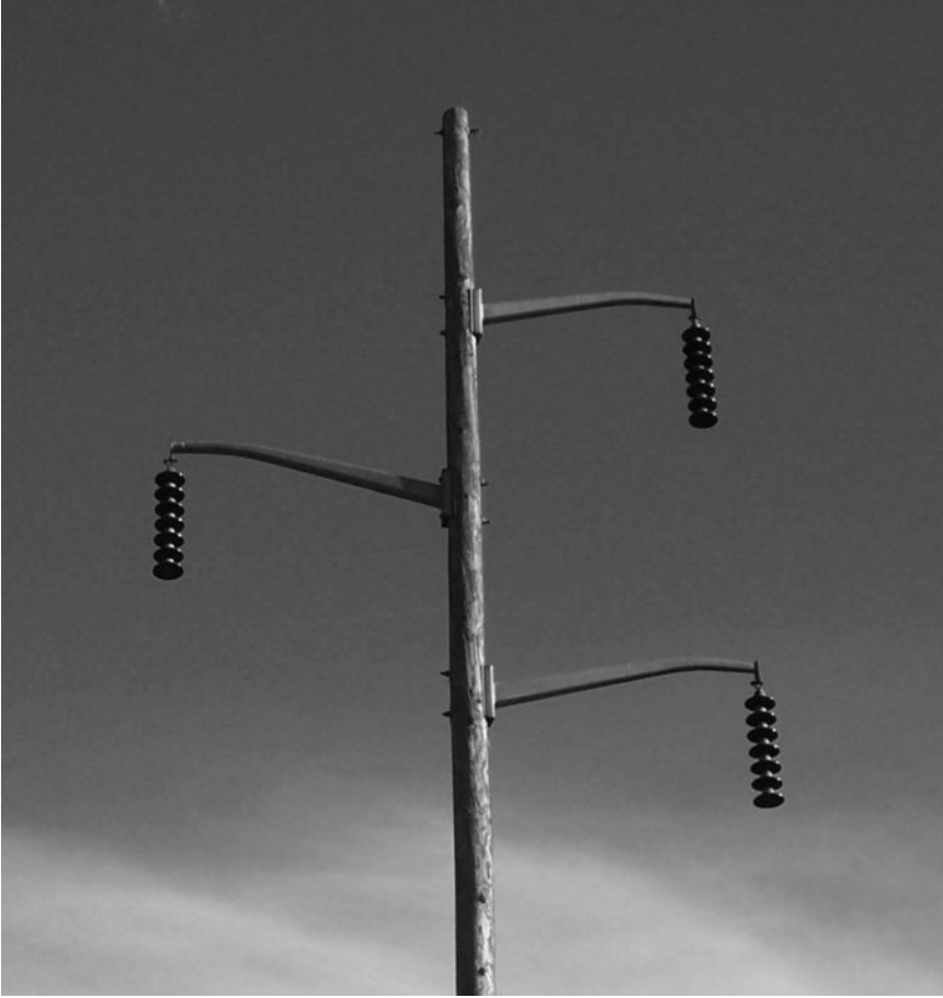
Figure 1.3b Wood Pole with Steel Davit Arms.
