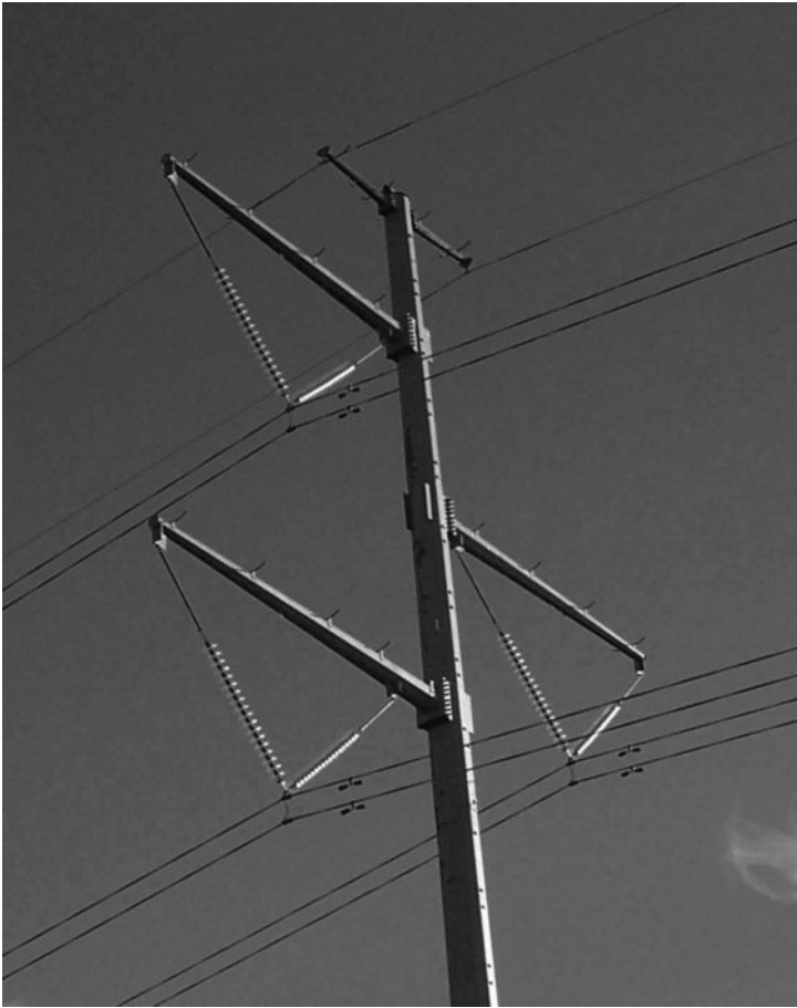
Figure 1.4a Steel Pole with V-String Insulators.
